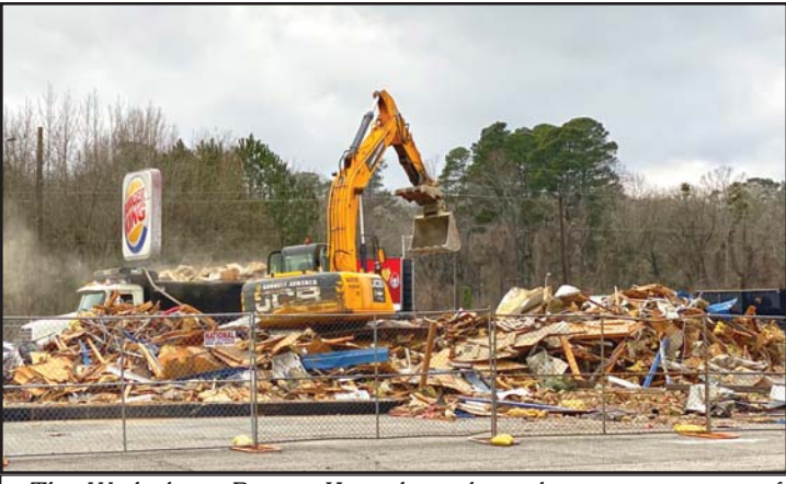
The Wadesboro Burger King drive-through is currently out of order. This photo of the demolition was taken on Tuesday, January 7.
