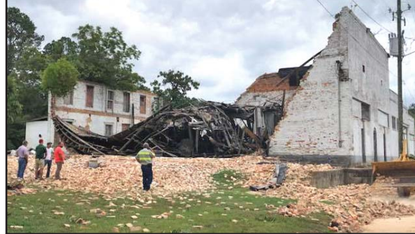
The former Polkton Shirt Factory building collapsed.
