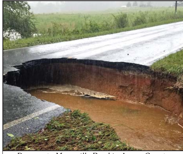
Damage to Mayesville Road in Anson County.
